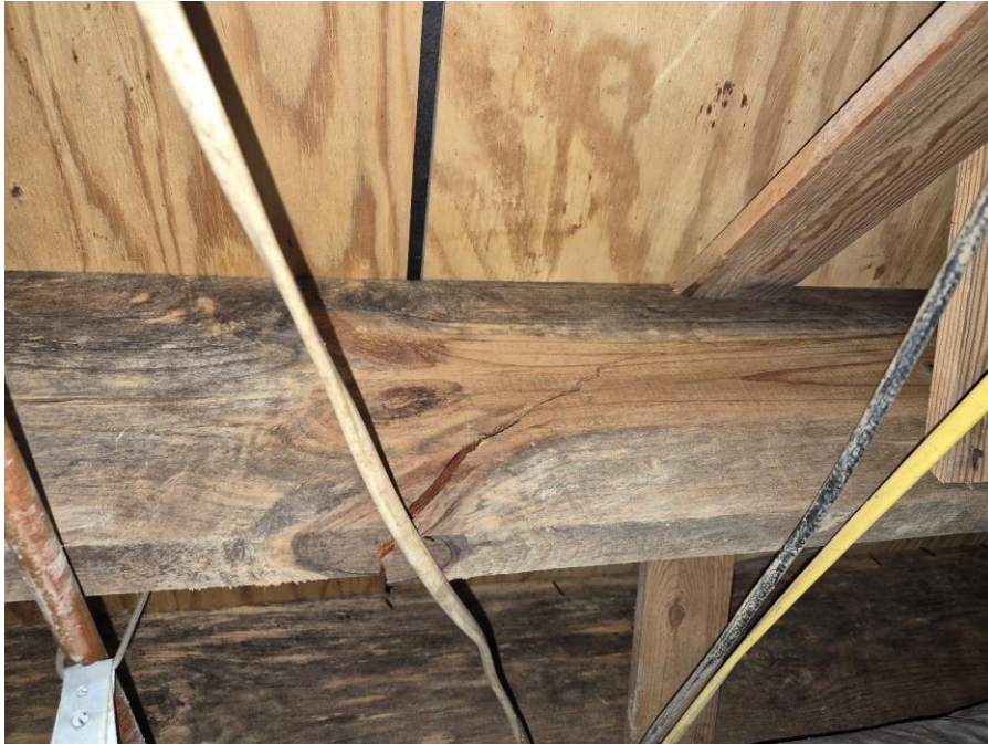
Picture 5 – Cracked joist
