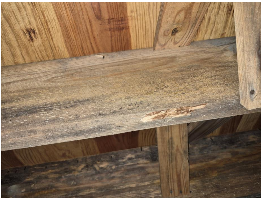
Picture 2 – Deteriorated joist
