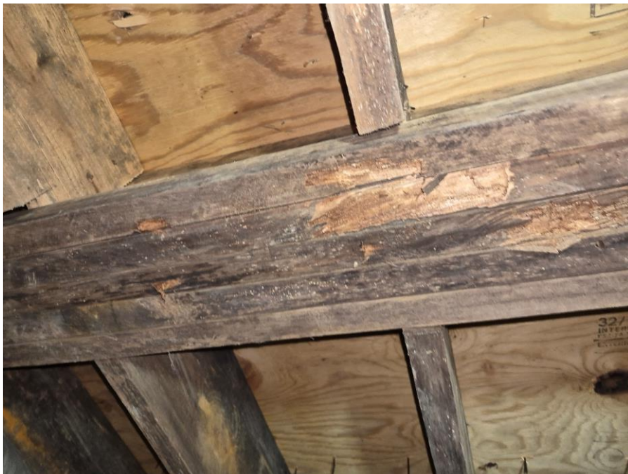
Picture 6 – Minor deteriorated girder
