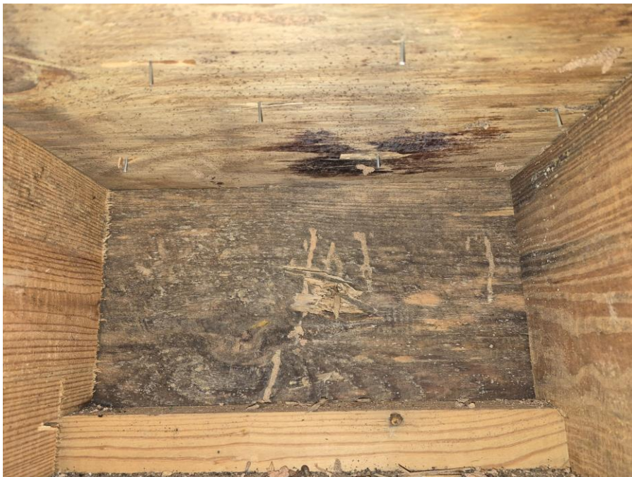
Picture 4 – Deteriorated rim beam
