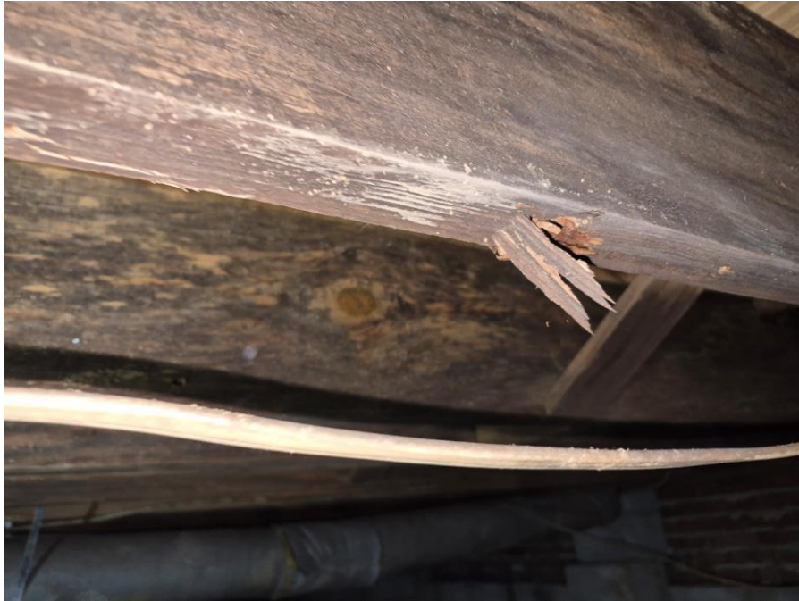
Picture 3 –Deteriorated joist
