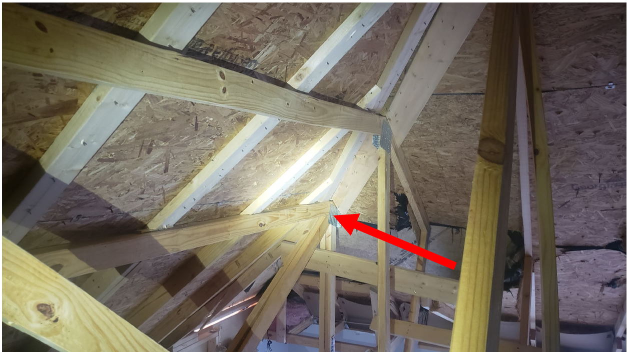
Item 1a) Girder truss to be repaired
