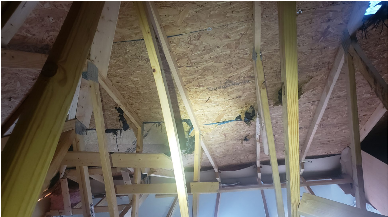
Examples of damaged trusses/areas to be repaired
