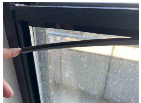
Noted at Bedroom #2
