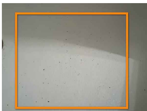
Noted at Hall Bathroom
