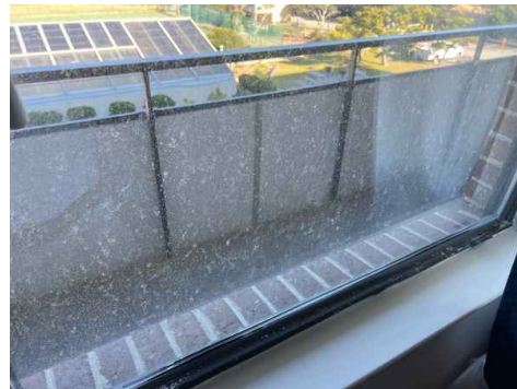
Noted at Bedroom #4
