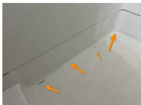
Noted at Hall Bathroom
