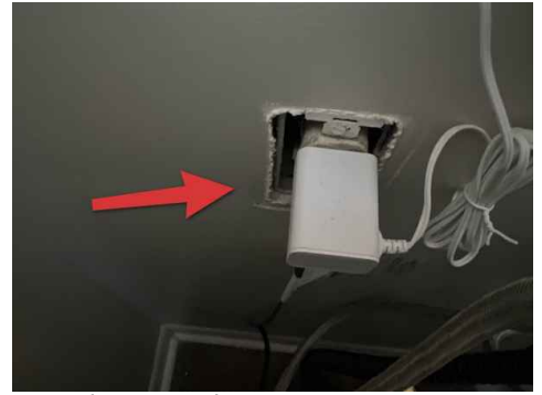
Noted at Laundry Room/Area
