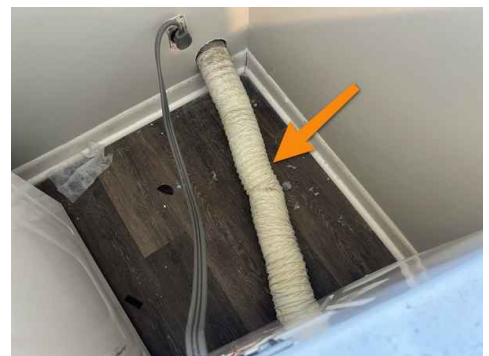
Noted at Laundry Room/Area
