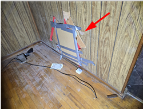
Damaged left rear Living room wall, adjacent to the kitchen.
