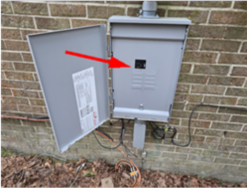
View of main electrical service disconnect on right side of home, cover on.
