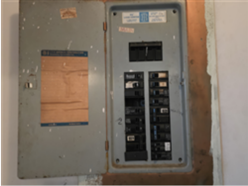
View of main electrical service panel in laundry room, cover on.
