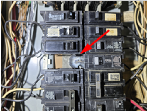
Knockout plug on the interior electrical panel cover is exposing a main bus bar that feeds a branch circuit is damaged. This condition indicates a history of arcing and or overheating. This condition presents a safety hazard that could result in interrupted service, property damage, and serious personal injury. A licensed electrical contractor should be consulted for repair and a complete evaluation of the electrical system.
