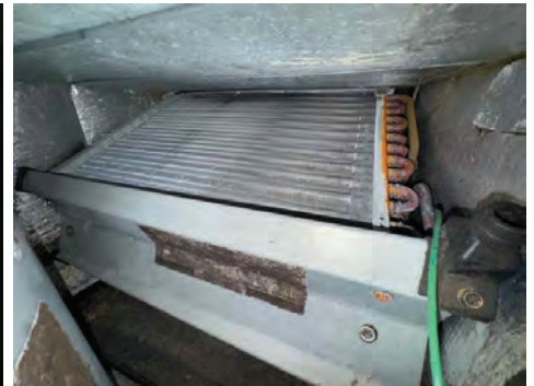
Front Right Eaves Air Handler Coil
