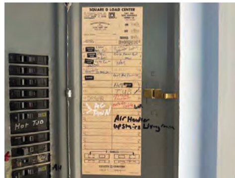
Hallway Main Panel
