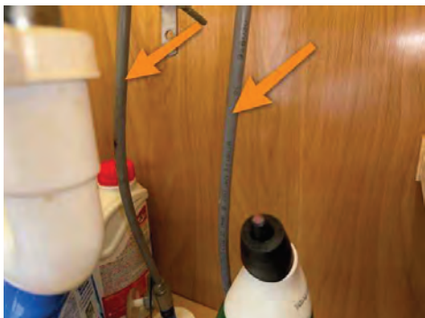
1st Floor Left Bathroom Sink
