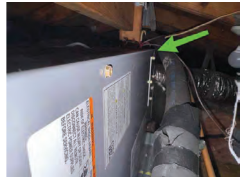
Attic Air Handler
