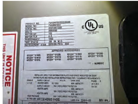
Front Right Eaves Air Handler Data Plate
