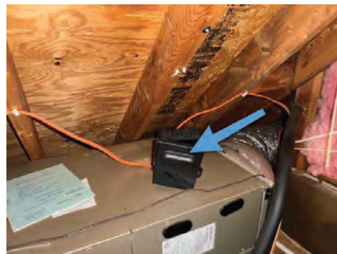
Front Right Eaves Air Handler
