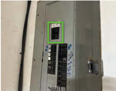
Garage Main Electric Disconnect
