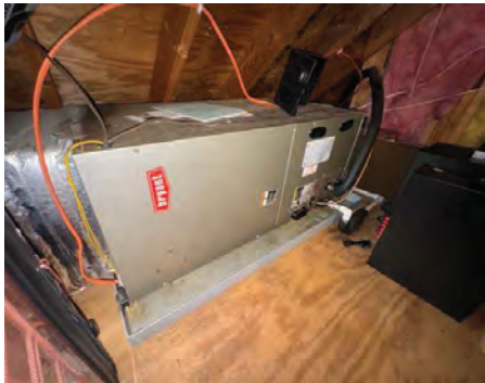
Front Right Eaves Air Handler
