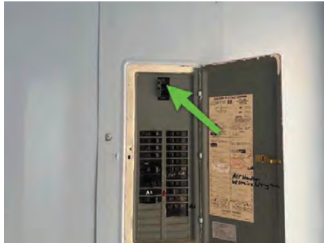
1st Floor Hallway Main Panel
