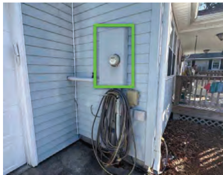
Electric Service Entrance
