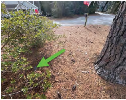
Main Water Shutoff
