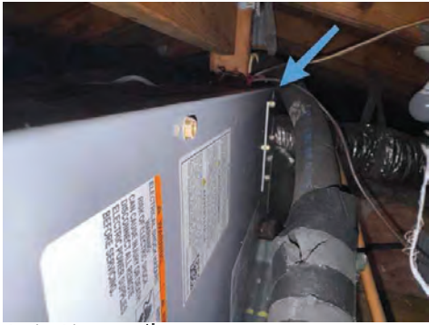
Attic Air Handler
