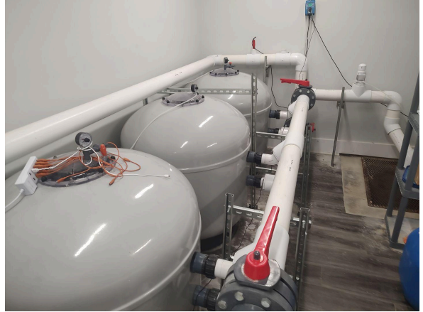
Pool pump equipment
