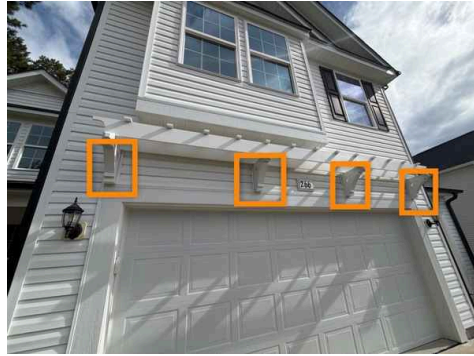
Front J channel to wood transition - gaps in sealant
