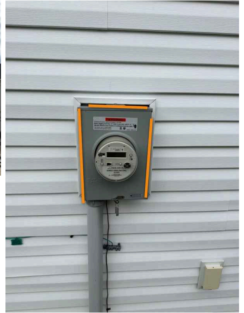
Right - J channel to meter transition
