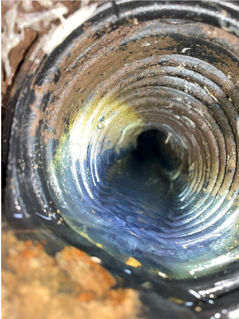
This picture shows water going down the only line that functions.
