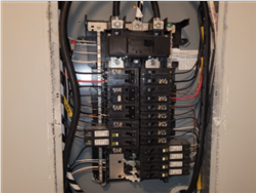
The electrical panel is in the laundry room, FYI.
