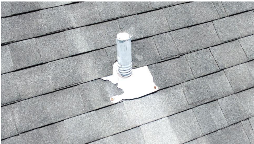
View showing damaged flashing for one of the plumbing vent pipes on the right roof slope.
