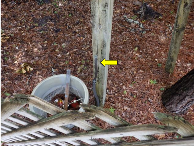
View showing the gas piping at the rear exterior. This has not been properly capped off and a regulator is not present.
