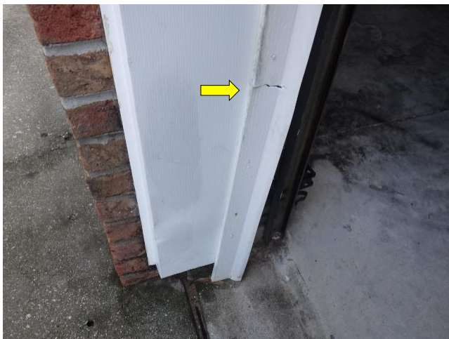
Weather stripping is damaged along the left side of the rear garage door and has been re-nailed into place. Replacement of this weatherstripping section is warranted to properly mate with the garage door when closed.
