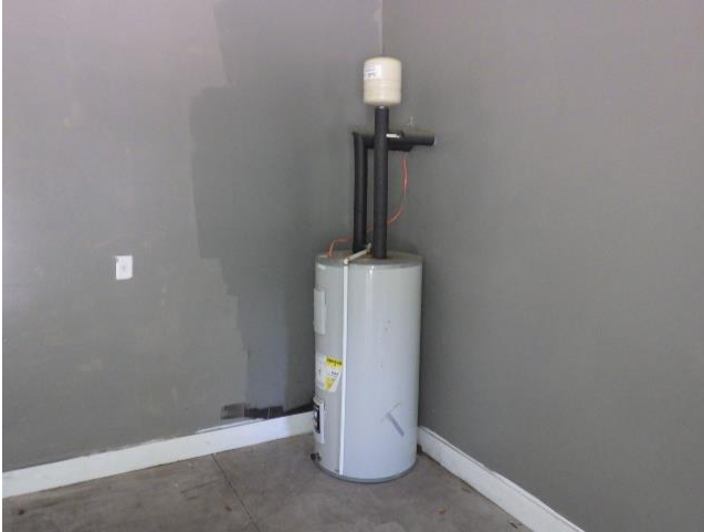
View showing the water heater in the garage.
