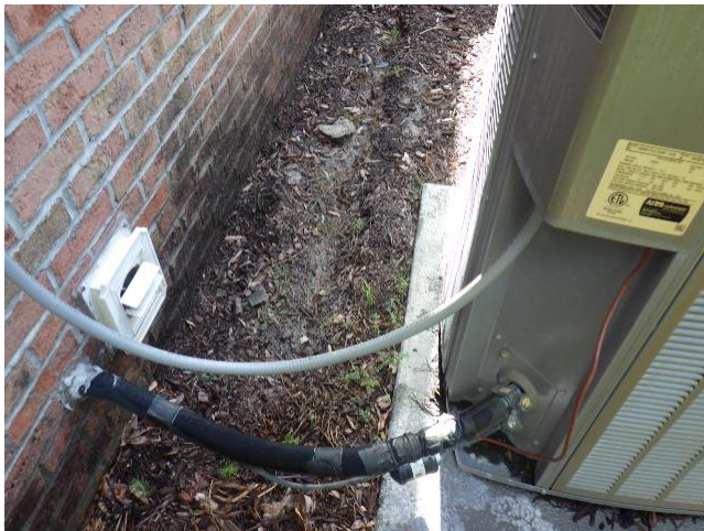
The dryer exhaust discharges at the right exterior directly behind the heat pump unit. This is not a desired condition as it could contribute to lint accumulation on the coil. Routine cleaning of this heat pump unit should occur due to this condition. Consider investigating possible relocation of the dryer exhaust hood through a qualified contractor.
