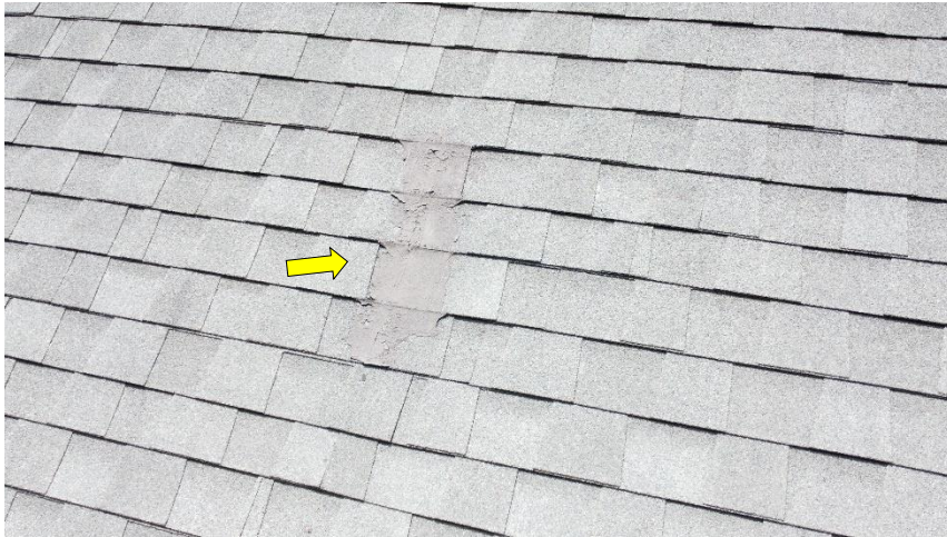
View showing roofing sealant applied to shingles on the rear roof slope. This is at an area where one of the dark stains observed from inside the attic.
