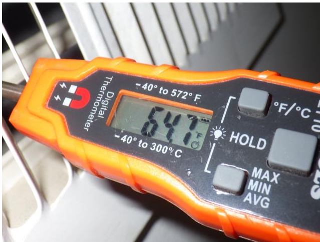
View showing a 64 degree cooling temperature produced at an air supply register for the zone 2 heat pump system.
