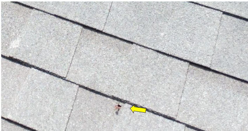
View showing a nail that has cut through the shingles on the rear roof slope. This is at an area where one of the dark stains is observed from inside the attic.
