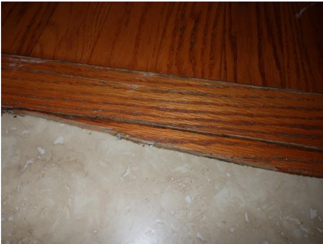
The transition strip between the foyer tile floor and wood flooring is partially cracked and missing. Replacement of this component is warranted.
