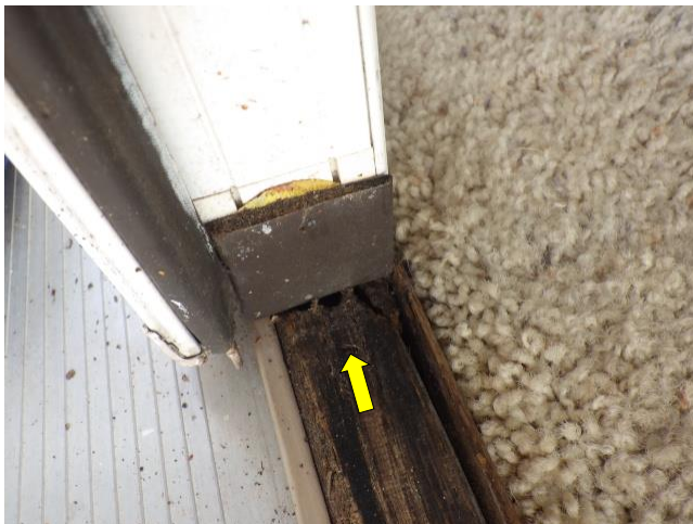
View showing water damage in the wooden component of the threshold where the secondary door latch bolt engages.
