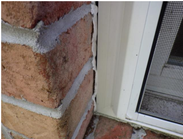
Second view showing caulking open along a window frame.
