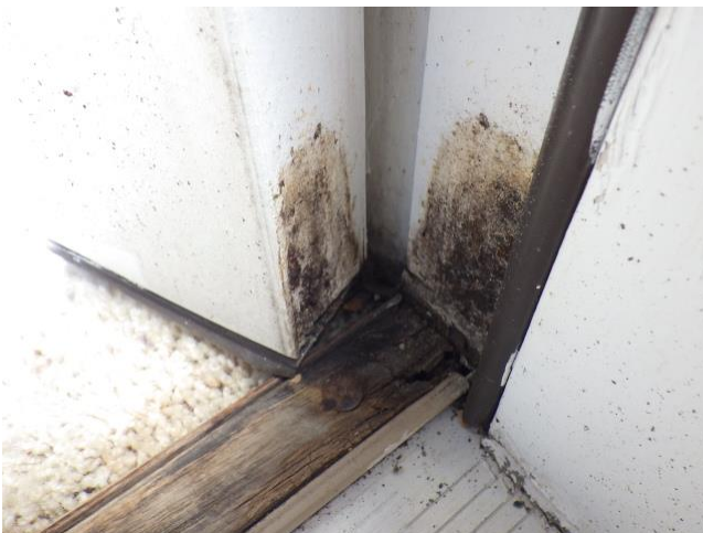
There is water damage in the trim and casing at the bottom corners near the threshold for the rear exterior double door unit at the primary bedroom. Additional water damage is visible at the bottom latch and hinge sides of this door unit (visible only with the doors open). Water damage is also present along the wooden threshold strip. Recommend investigating these conditions further through a qualified contractor and repair/replace these components as needed.
