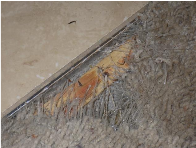
There is a small area of damaged carpet at the entry leading into the primary bathroom. Placement of this carpet section is warranted.
