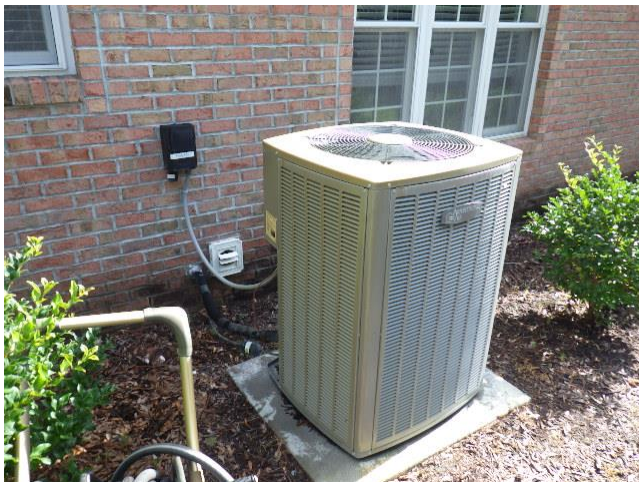
The right exterior heat pump unit exhibits a significant amount of movement on its pad when pressure is applied (rocks back-and-forth). Recommend investigating action through a qualified HVAC technician to install shims or other modification to fully stabilize the unit.
