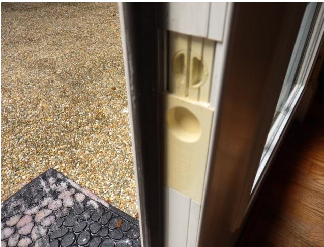
View showing the bottom latch bolt mechanism for the secondary door for the living room exterior door unit that will not release with reasonable effort. This door cannot be operated due to this condition and additional damage may exist that is not identified in this report.
