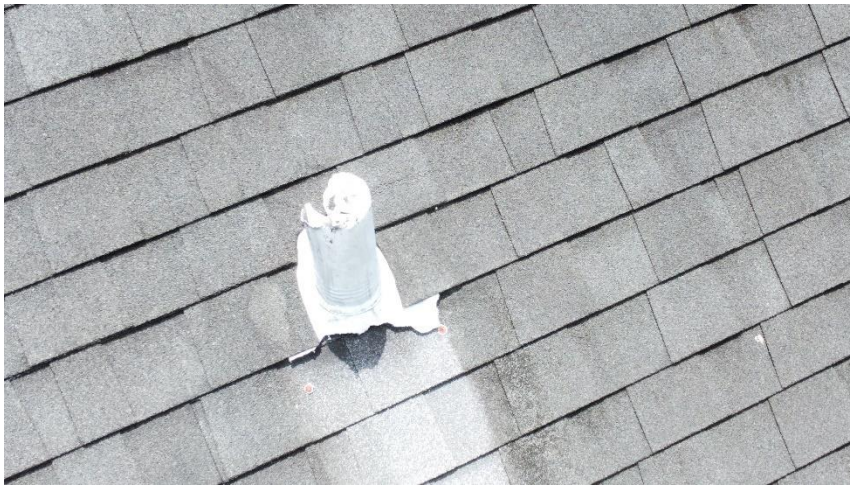
View showing damage to flashing for the plumbing vent pipe on the left roof slope. The vent pipe itself is also damaged from possible squirrel activity. Replacement of this vent pipe section appears warranted during shingle and flashing replacement. This may involve cutting the pipe from inside the attic and splicing in a new section.
