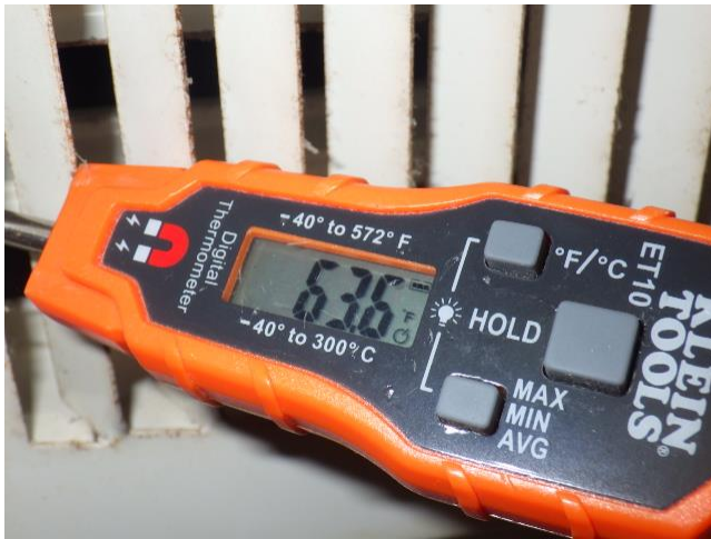
View showing a 63 degree cooling temperature produced at an air supply register for the zone 1 heat pump system.
