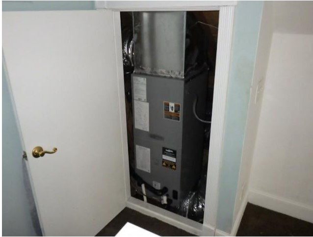
View showing the FROG air handler.
