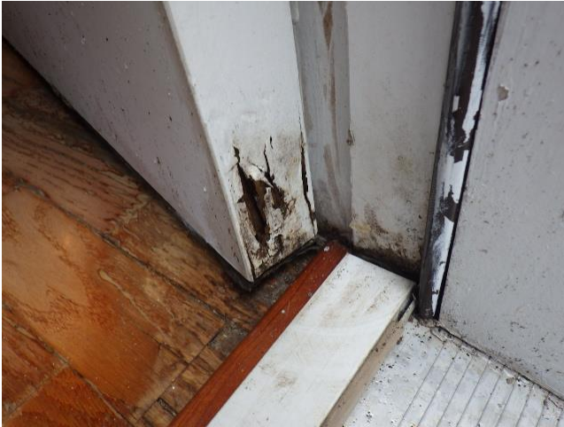
View showing water damage at the bottom hinge side of the main door.
