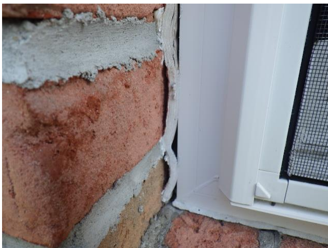
Caulking has opened at many of the windows around the building's exterior where the frames meet the brick veneer. Action is warranted to clean away the old caulking, then re-caulk to seal the frames with the brick veneer.
