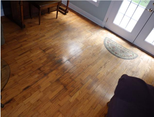
View showing flooring in the living room that is weathered and stained.
