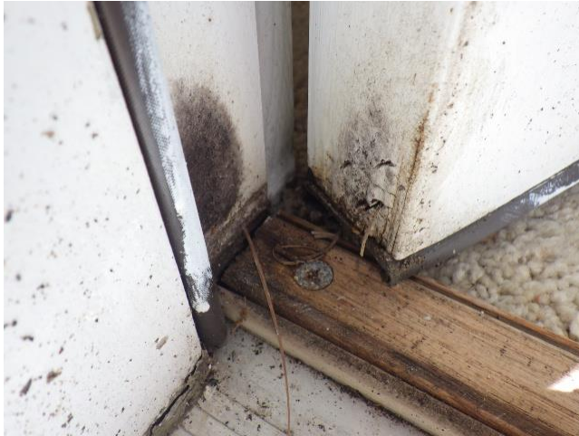
View showing minor water damage at the bottom hinge side of the secondary door for the double door unit at the primary bedroom.
