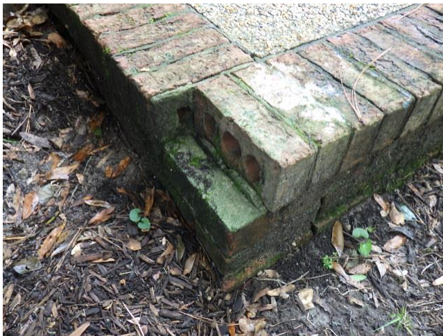
One brick is missing at the outer corner of the rear concrete patio. Installation is warranted through a qualified contractor.
