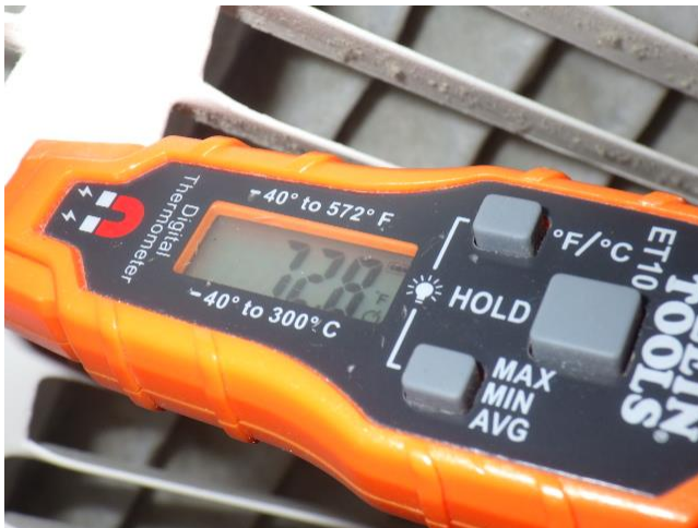
View showing the 72 degree temperature produced at a central air return for the zone 1 heat pump.
