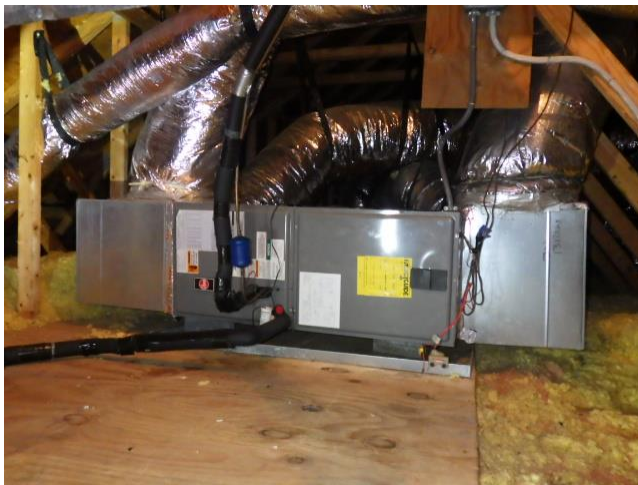
View showing the high attic air handler.
