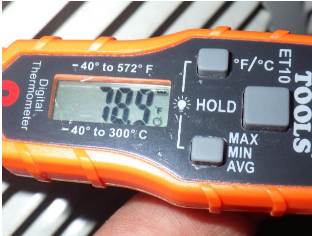
View showing the 78 degree temperature produced at a central air return for the zone 2 heat pump.
