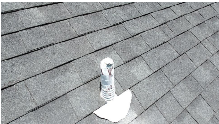
View showing damaged flashing for the second plumbing vent pipe on the right roof slope.
