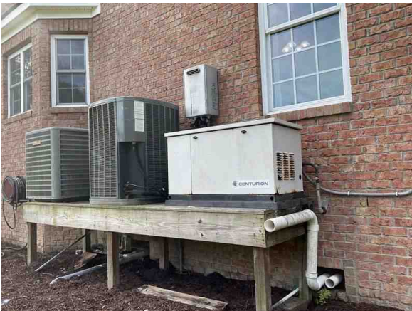
A/C Units Generator
