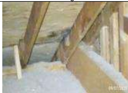
Moisture Stains at Front Right Sheathing
