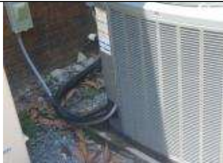
Deteriorated Refrigerant Line Insulation
