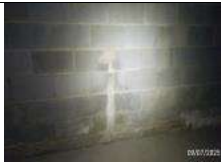
Efflorescence at Rear Left Foundation
