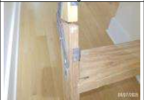
Right Pull Down Stairs Hardware Damaged
