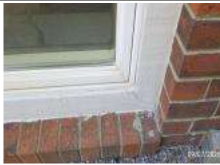
Cracked Trim at Front Center Left Window
