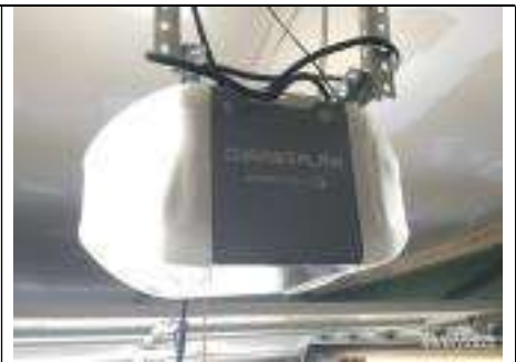
Garage Door Opener
