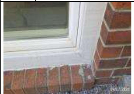
Cracked Trim at Front Center Left Window
