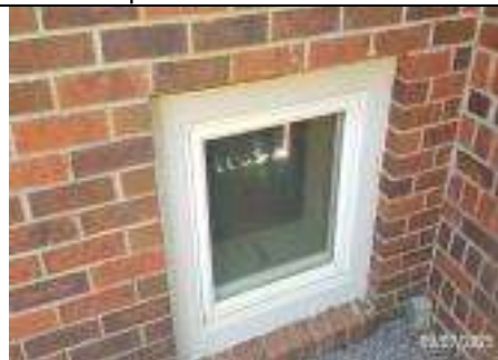
Cracked Trim at Front Center Left Window
