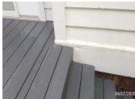
Deteriorated Trim at Rear Left
