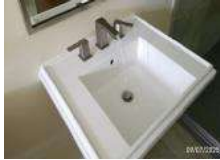
Inoperable Drain Stopper at Master Right Sink
