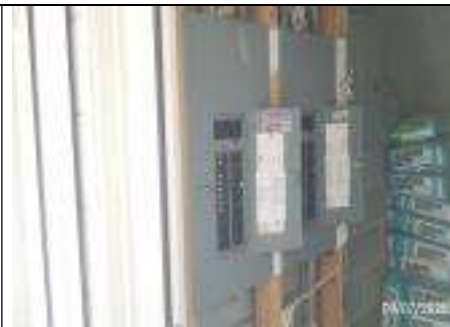
Main Electric Panels
