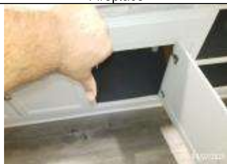
Lower Disposal is Inoperable
