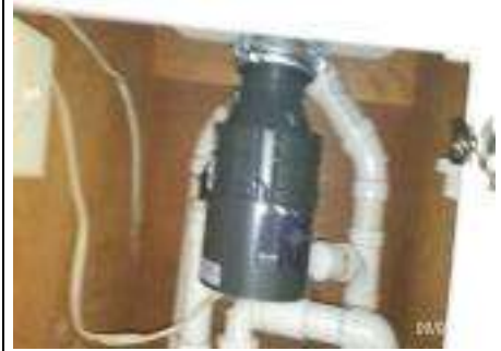
Lower Disposal is Inoperable
