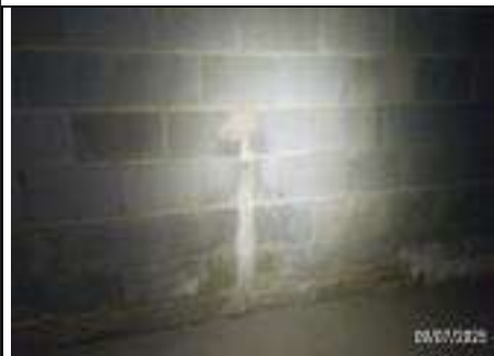
Efflorescence at Rear Left Foundation
