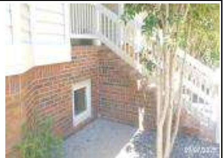
Cracked Trim at Front Center Left Window
