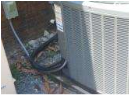
Deteriorated Refrigerant Line Insulation
