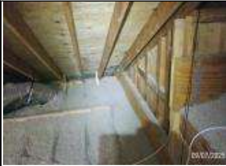
Moisture Stains at Front Right Sheathing
