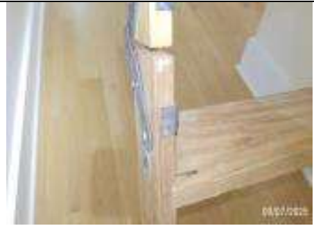
Right Pull Down Stairs Hardware Damaged
