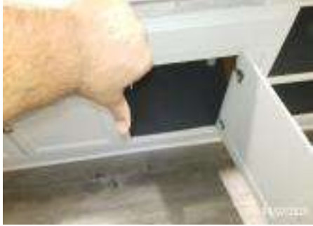
Lower Disposal is Inoperable
