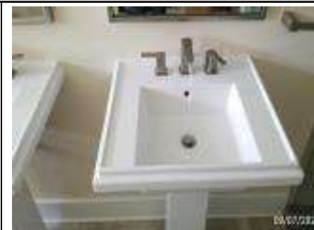
Inoperable Drain Stopper at Master Right Sink
