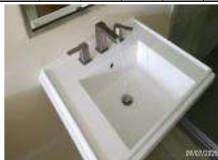
Inoperable Drain Stopper at Master Right Sink
