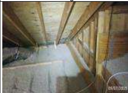
Moisture Stains at Front Right Sheathing
