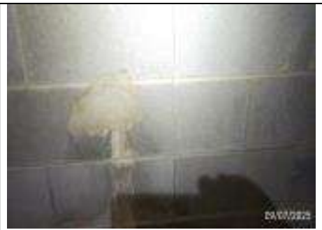
Efflorescence at Rear Right Foundation
