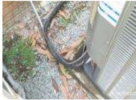
Deteriorated Refrigerant Line Insulation
