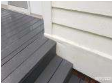
Deteriorated Trim at Rear Left
