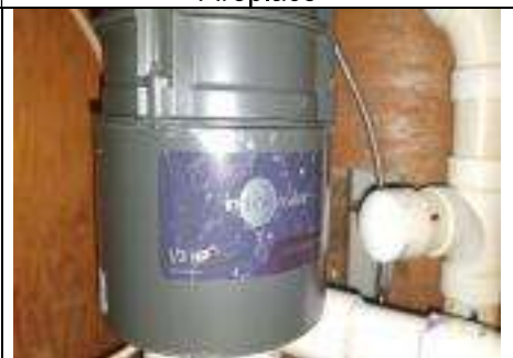
Lower Disposal is Inoperable
