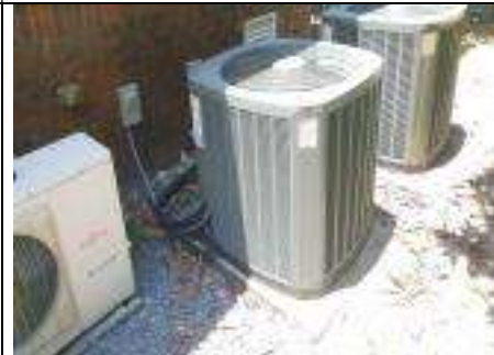
Heat Pump Equipment
