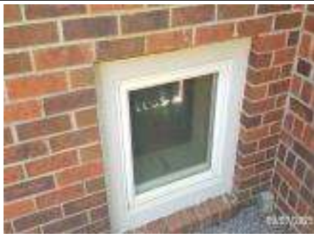
Cracked Trim at Front Center Left Window
