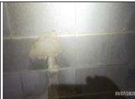
Efflorescence at Rear Right Foundation
