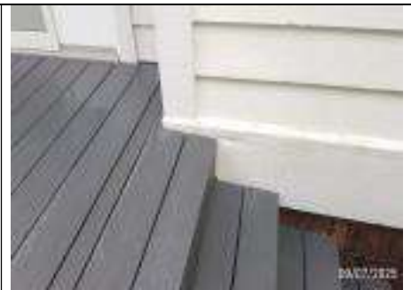
Deteriorated Trim at Rear Left
