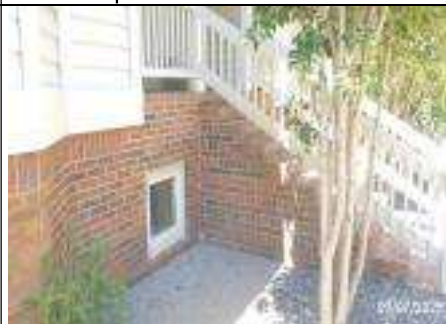
Cracked Trim at Front Center Left Window
