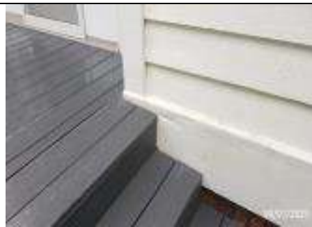
Deteriorated Trim at Rear Left
