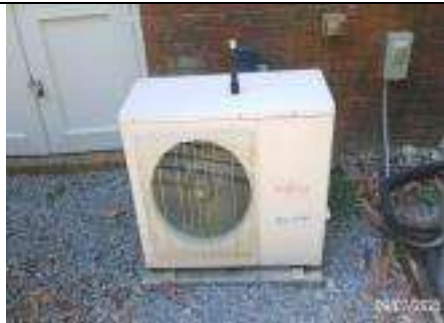
Heat Pump Equipment
