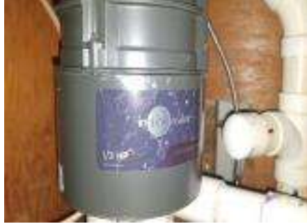
Lower Disposal is Inoperable
