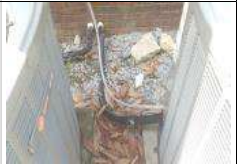
Deteriorated Refrigerant Line Insulation
