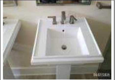
Inoperable Drain Stopper at Master Right Sink
