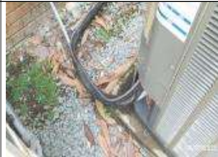
Deteriorated Refrigerant Line Insulation
