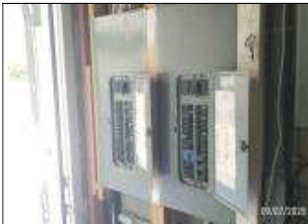
Main Electric Panels
