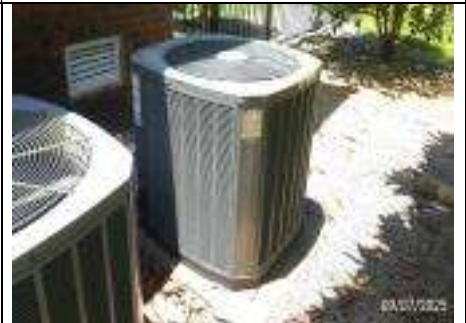
Heat Pump Equipment
