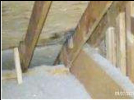
Moisture Stains at Front Right Sheathing
