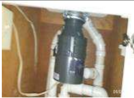
Lower Disposal is Inoperable
