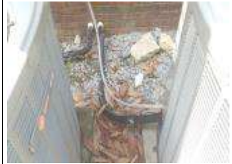
Deteriorated Refrigerant Line Insulation
