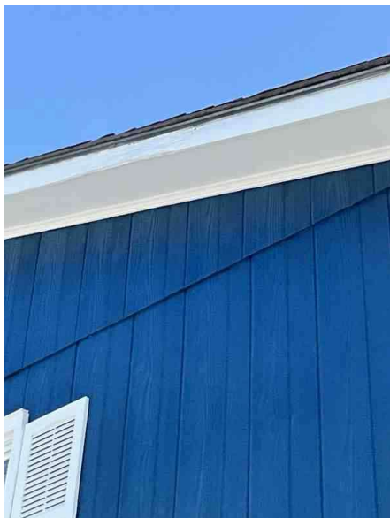
Replace damaged/decayed exterior woodwork
