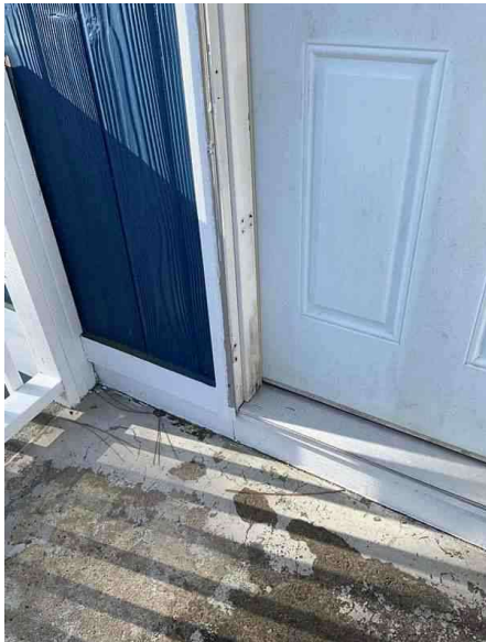
Replace damaged/decayed exterior woodwork
