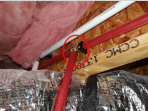
Additional photo showing corrosion on brass PEX fitting above the water heater.
