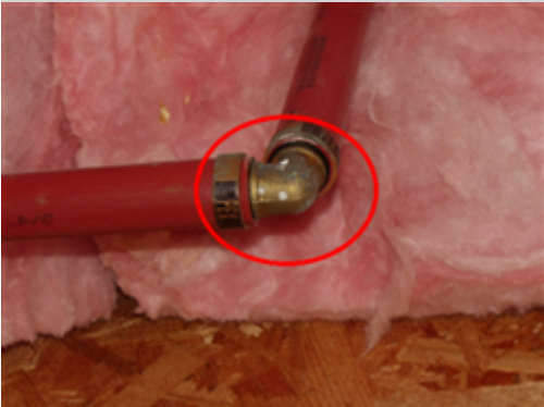
The visible plumbing lines in this home are cross-linked polyethylene (PEX) with brass fittings. Evidence of discolored/corroded fittings was noted during the basement inspection. This could be the result of dezincification of the brass alloy. Dezincification occurs when zinc leaches from the brass leaving the fittings in a weakened state. As the zinc leaches, it can also form a build-up inside the fitting restricting water flow and ultimately leaving the plumbing system prone to failure. A licensed plumbing contractor should be consulted for a complete evaluation of the plumbing system to determine the significance of this concern and to make necessary repairs.
