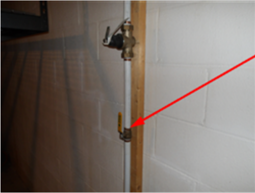
Photo showing emergency water shut off located in basement utility room area.
