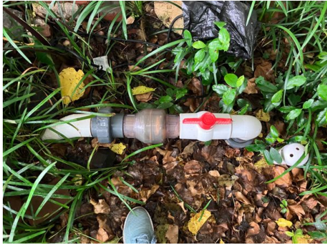
Sewage eject pump/lift station
