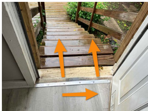
Door binds on floor/no landing for steps at exit.
