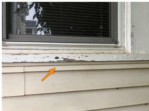
Peeling Paint Exterior wood trim
