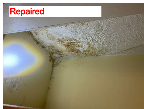
Patching/Stain in ceiling behind refrigerator
