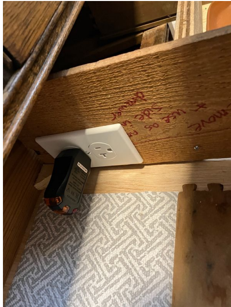
Master Bath sink base cabinet drawers- receptacle not connected to Power
