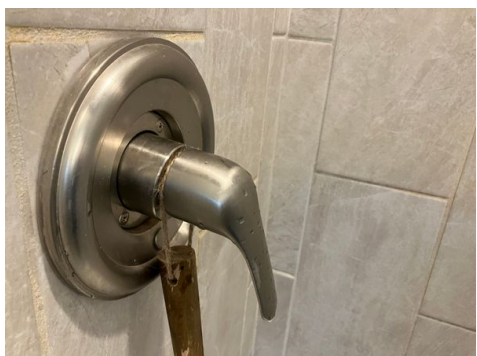
Right Side Bathroom Shower Control loose/unsecured
