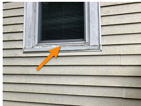
Peeling paint on exterior wood trim
