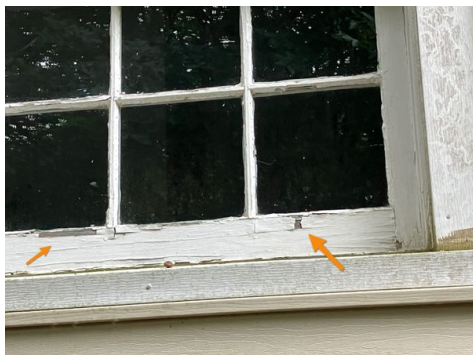
Window trim/cracked glazing compound
