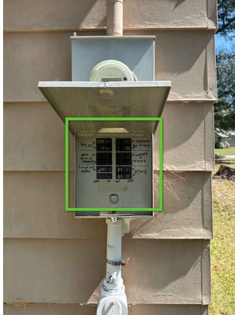
Throw all 6 breakers to disconnect all power
