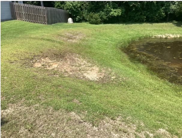
Minor shoreline erosion
