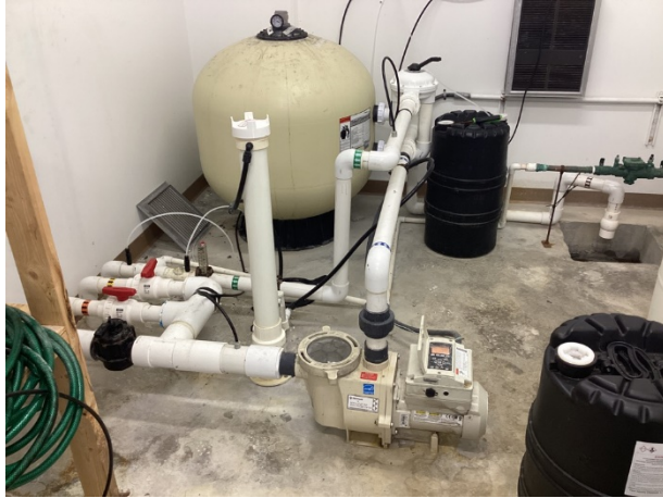
Pool pumps and filters
