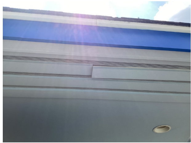
Wood soffit deterioration
