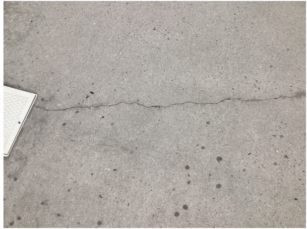
Isolated cracks evident
