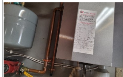
Recommend on demand hot water boiler be cleaned and serviced
