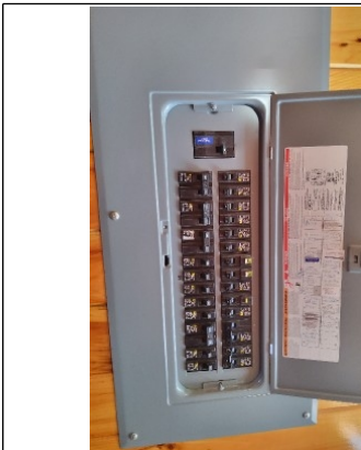
Main electric panel located in 1st floor hallway
