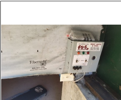
Septic tank high and low water alarm located in the basement bulkhead door
