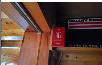
Emergency shut off switch located in the kitchen pantry
