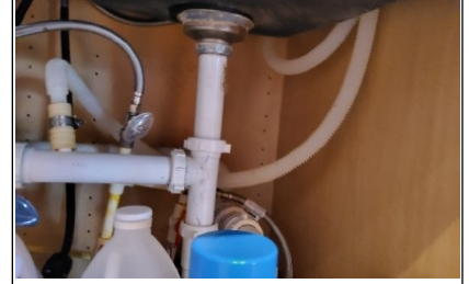
Dishwasher drain line is looped to prevent sink water from back flowing into the dishwasher
