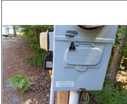
Install a lock on exterior meter disconnect panel door
