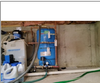
Water entrance along the north side of the basement
