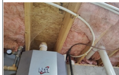
Intake and exhaust
