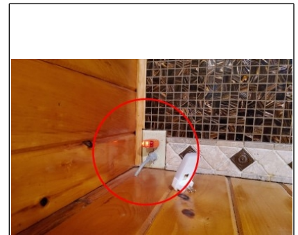
Outlet is GFCI protected, trips along south wall of the bathroom
