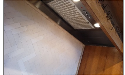
Exhaust fan is noisy
