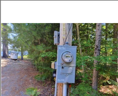
Meter located on the utility pole
