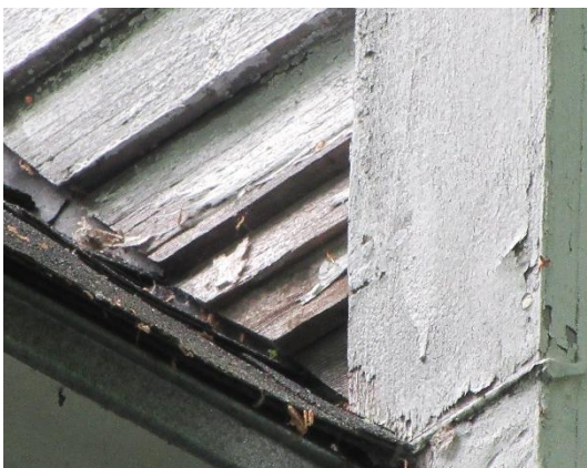
peeling siding paint
