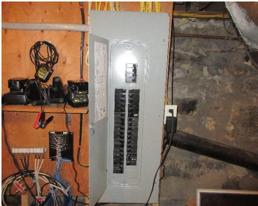
main breaker panel(s)
