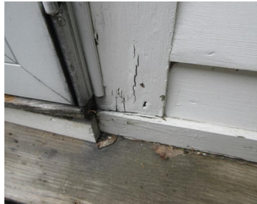
rot at lower door trim
