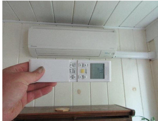
kitchen heat pump head unit
