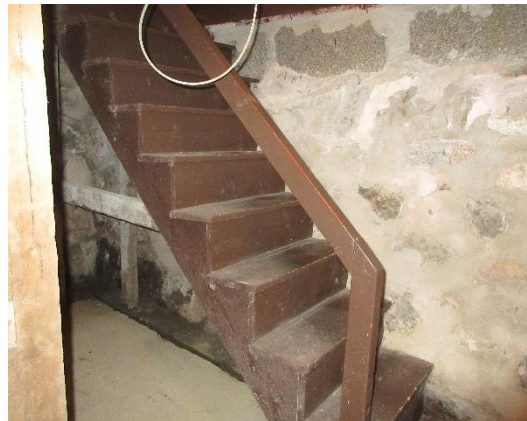
stairs lack adequate railings
