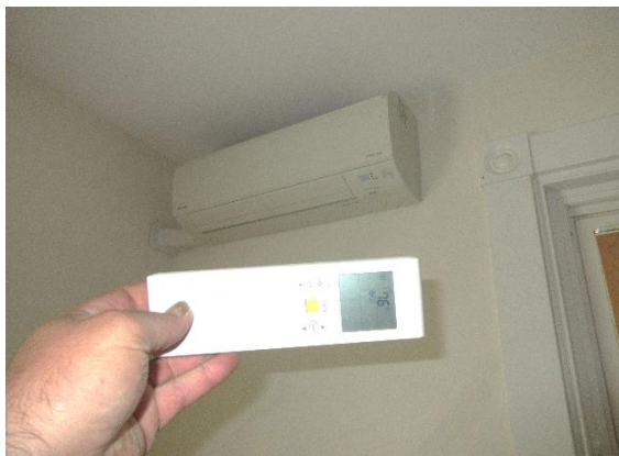
1st floor bedroom heat pump head unit
