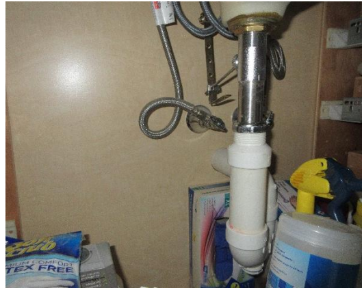
primary bath; plumbing under sink
