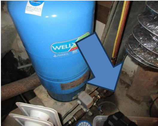
main water supply and main shut off valve at arrow
