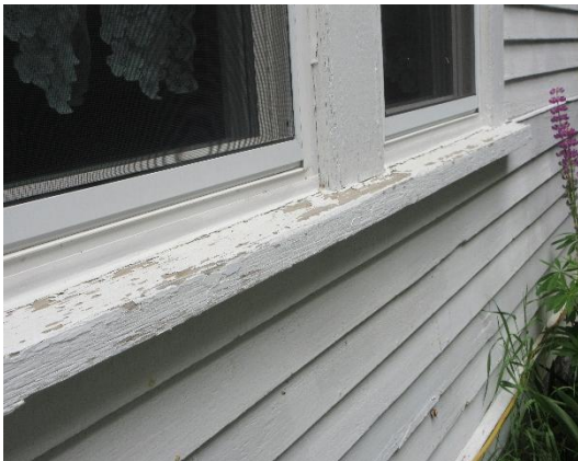
peeling paint at window sill, trim
