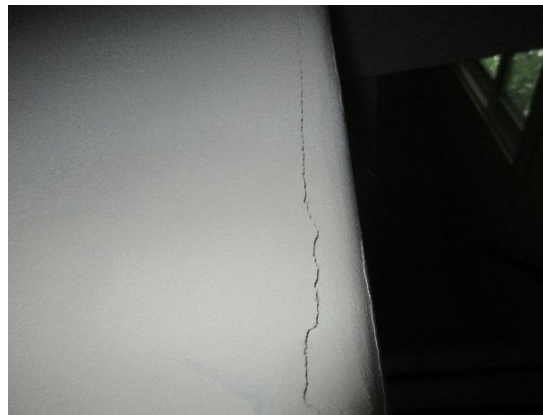
crack in plaster
