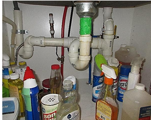
plumbing under kitchen sink
