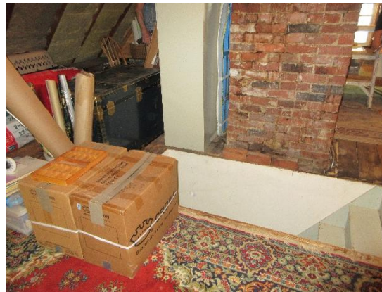
opening around top of stairs lack fall protection
