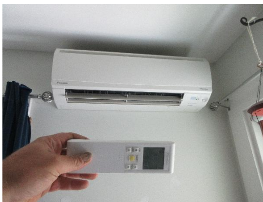
primary bedroom heat pump head unit
