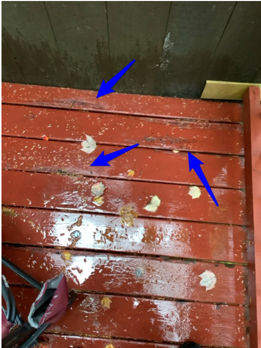
Areas of deterioration
