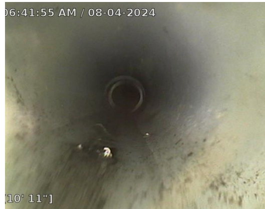
pipe to leach field
