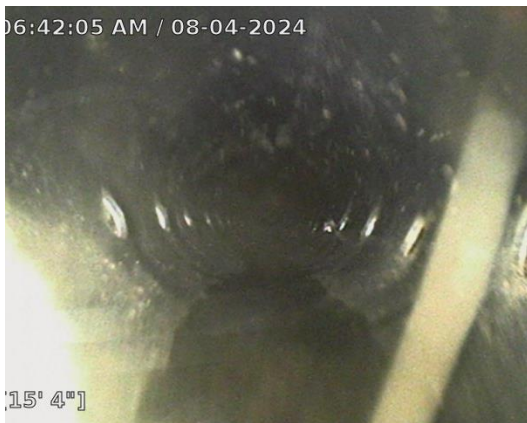
leach field piping
