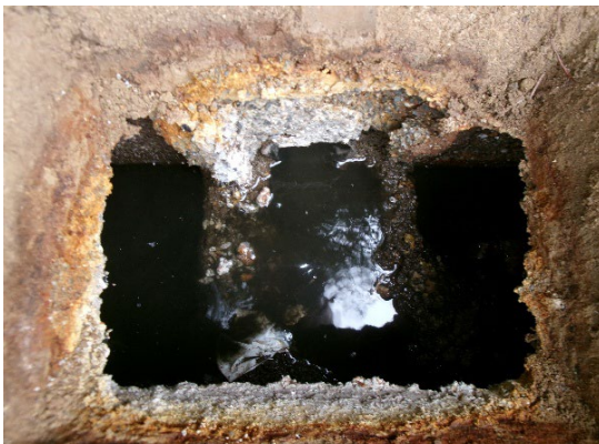
Outlet Cover and bad Baffle
