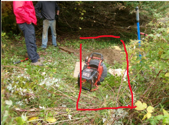
Septic Tank Location
