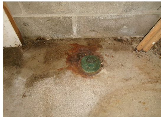
Piping From House to Tank
