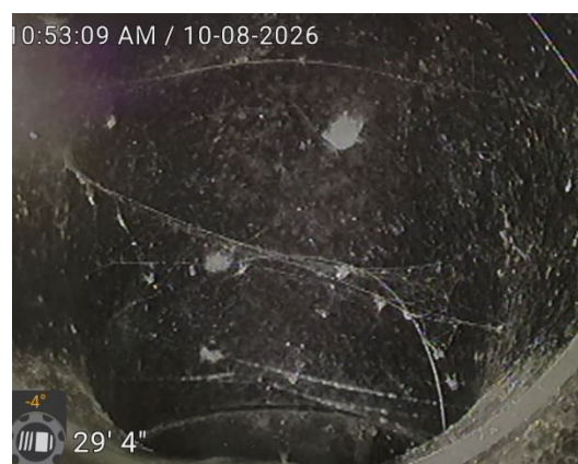
drop in pipe
