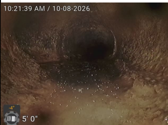
pipe from house to tank
