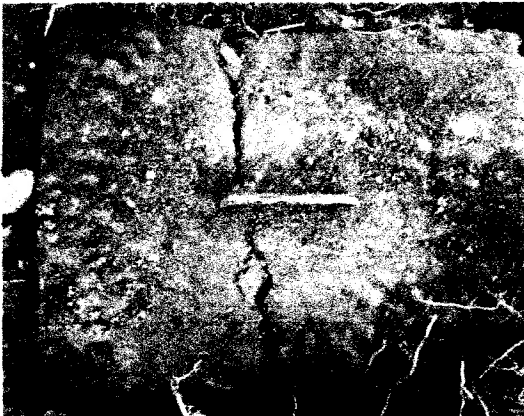
cracked outlet cover
