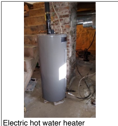
Electric hot water heater
