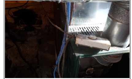
Furnace dehumidifier control has been discontinued
