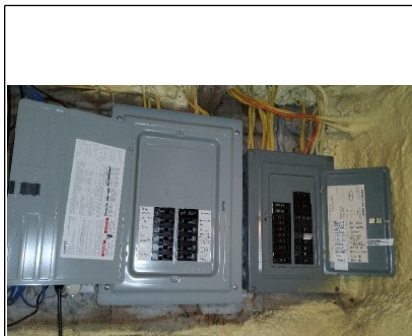
Main and sub panel in the basement
