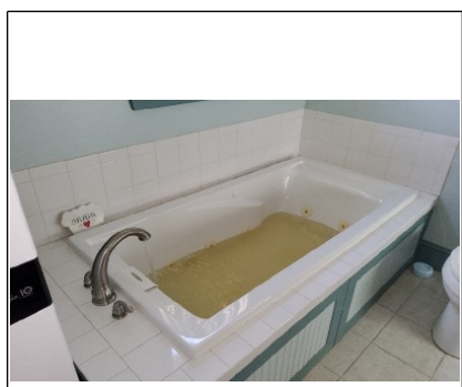
Jet tub Water is discolored. Hot water tank has not been used for awhile. Assure jet tub is on a GFCI protected outlet or breaker.
