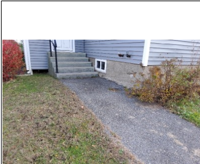
Walk way, some settlement observed
