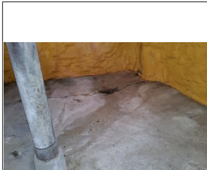
Filling cracks with a water plug cement may reduce water seepage into the basement
