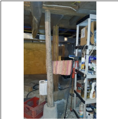
Recommend installing an additional steel column adjacent to east basement wood columns
