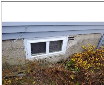
Repair damaged north concrete stem walls, concrete has chipped away
