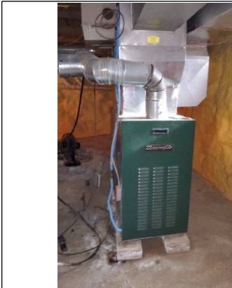
Oil,fired forced hot air furnace
