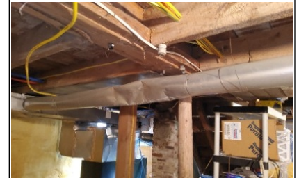
Some ductwork is dented
