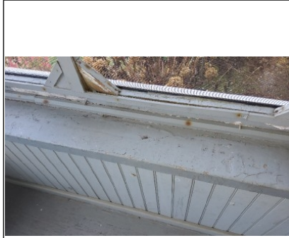
Chipping and peeling paint. Homes of this age may contain lead base paint. Maintain painted surfaces to minimize lead paint exposure
