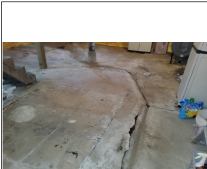
Concrete slab, hummed in the center to divert water seepage toward the sump pump
