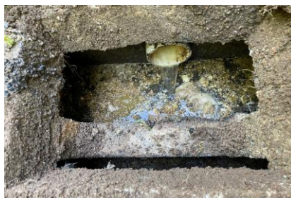
schedule 40 PVC inlet pipe & concrete splash-plate baffle
